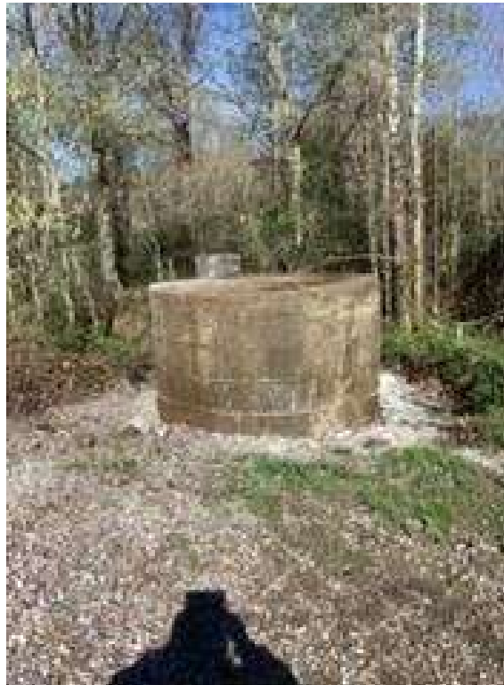
Manhole 1865 - 352 Fontana Road After Cleanup
